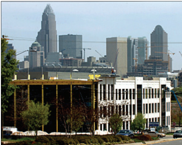
DAVIE HINSHAW / Staff Photographer 4/09/08 - The Charlotte School of Law, under construction at Suttle Avenue and Wilkinson Boulevard.
